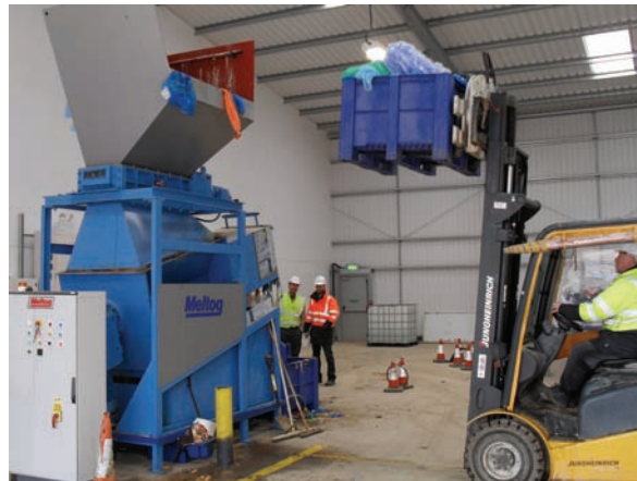
Packaged waste food taken in Dolav to depacking equipment
